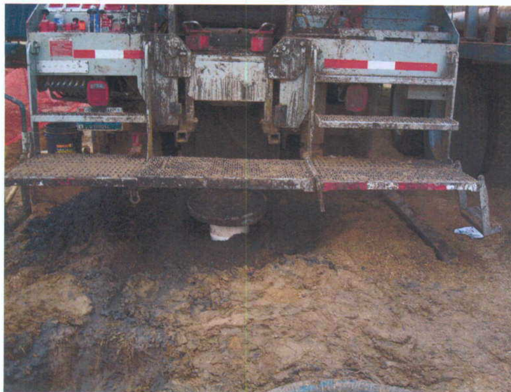
Photo #6: Hole covered, west site
